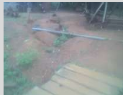
Plate 1: Exposed water supply pipelines due to severe erosion..
