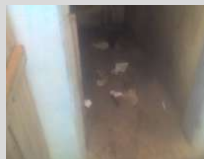
Plate 3: : Faecal matter floor of privy rooms.
