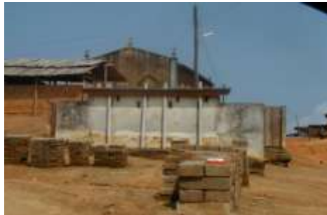
Plate 2.6: Communal Toilet showing erosion of around the base of superstructure
