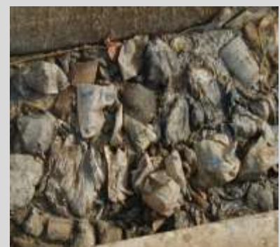
Plate 2.3: Storm drain heavily choked with plastics containing excreta
