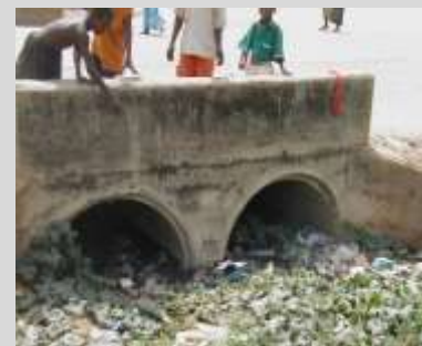
Plate 2.4 Cross culvert heavily silted with solid waste, Mankessim
