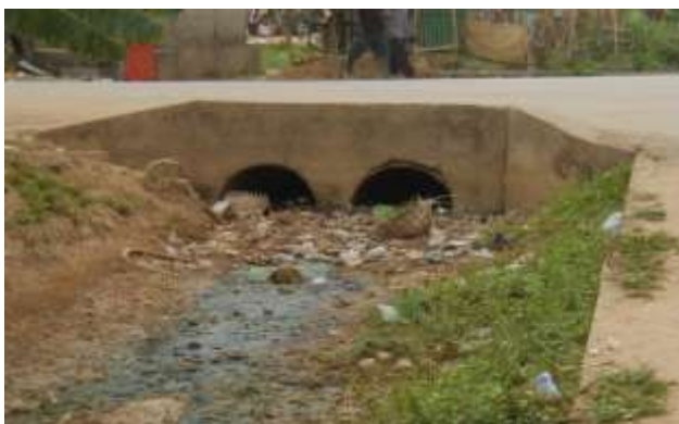
Plate 2.7: Circular culvert heavily silted with solid waste
