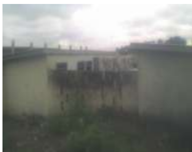
Plate 12: Old dilapidated 12 seater KVIP.
