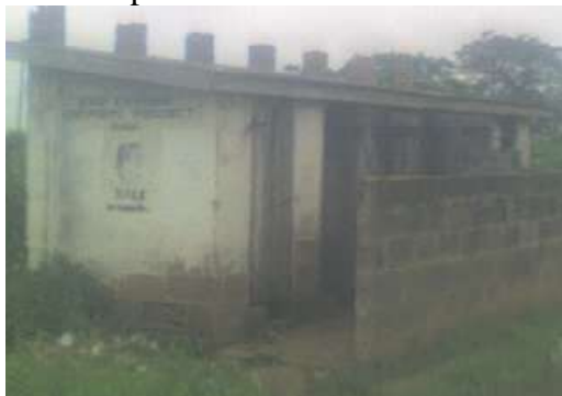
Plate 8: Old dilapidated 6 seater KVIP
