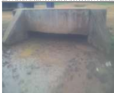
Plate 14: Heavily silted box culvert.
