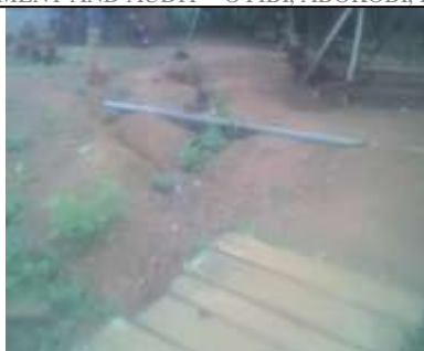
Plate 15: Exposed water supply pipelines due to severe erosion..
