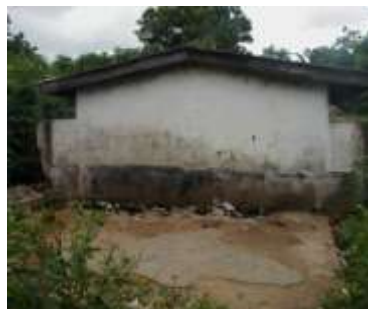
Plate 5: Old dilapidated 20 seater KVIP, Asutsuare.
