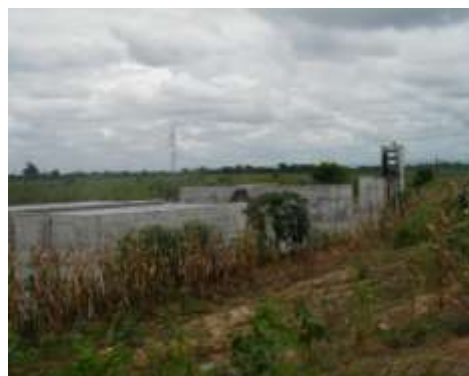
Plate 2: Water Treatment system for the newly constructed Osudoku Area Water Supply Scheme, Asutsuare
