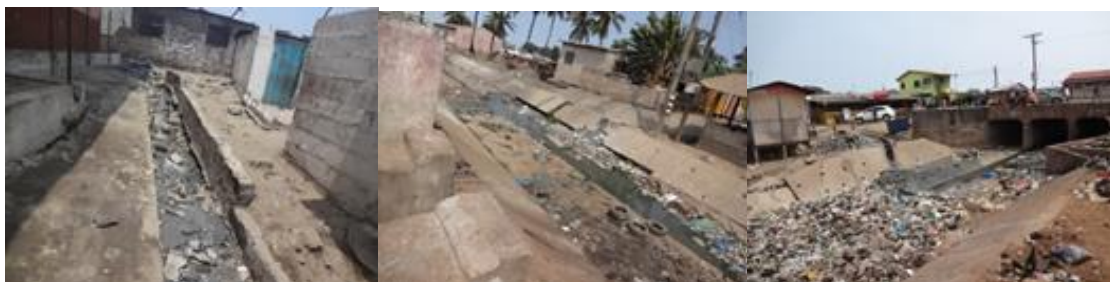
Plate 2-5: Drains in community silted with solid waste
