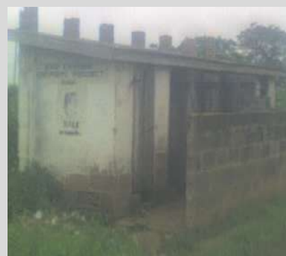
Plate 2: Old dilapidated 6 seater KVIP
